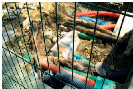
Underground services, one of the constraints found with urban planting
